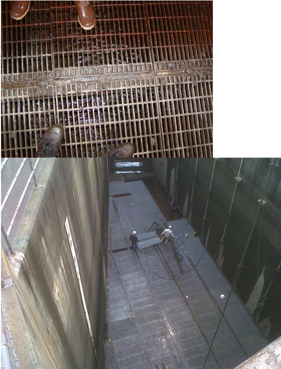
Figure 4: Diffuser gratings and flat bars being installed at The Dalles Dam. [Photo credit: Robert Cordie, US Army Corps of Engineers]
